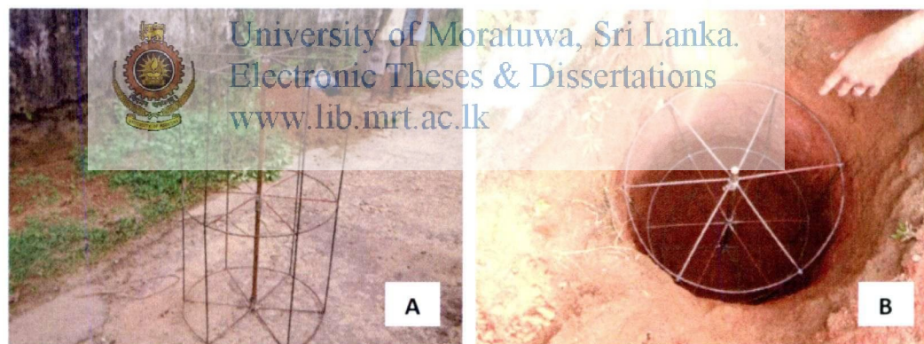
Figure 2.3 : Concrete Mesh Earth (A) Mesh before concreting, (B) Mesh inserted into the ground pit before concreting (Original is in colour)
